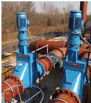
An inline TASKMASTER TM1630-18 being fed by an 18" force main.
